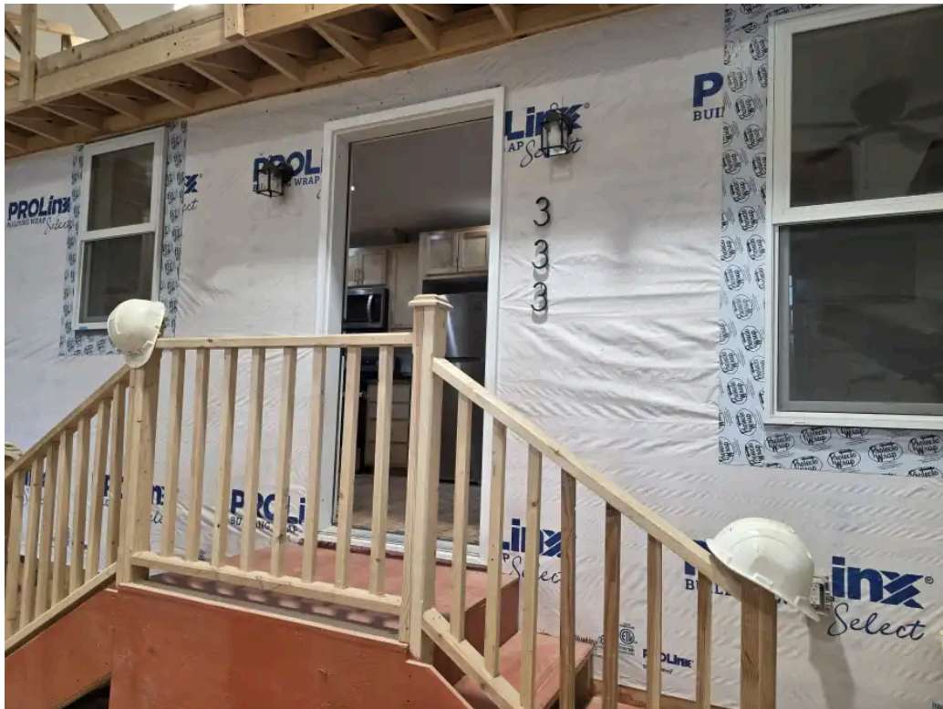
Students in architecture, carpentry, plumbing, electrical and HVAC planned and built a functioning house inside the school's massive carpentry lab.
