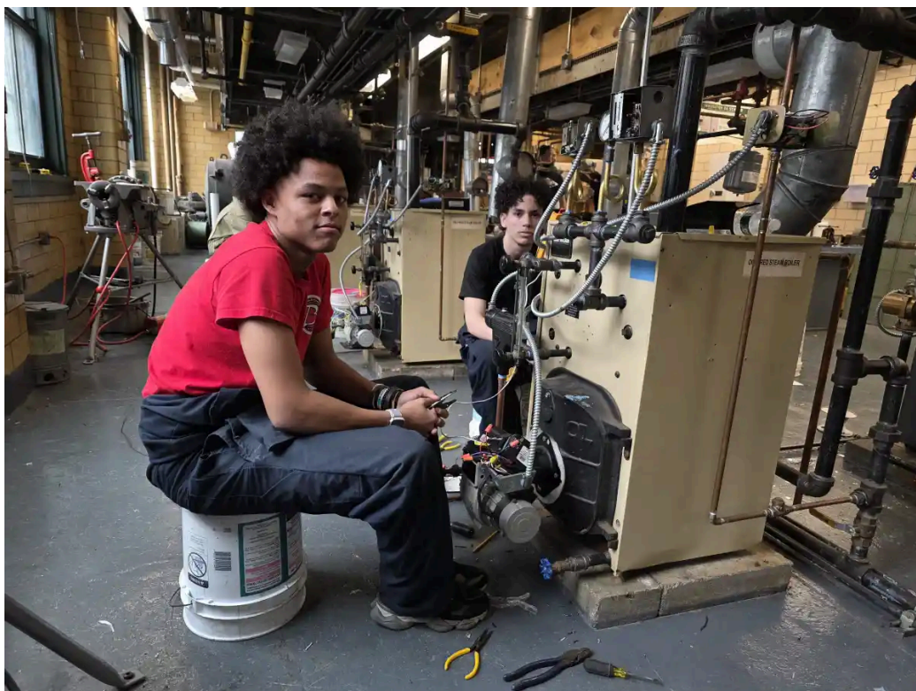
José Germosen and Ryan Nunez are both juniors studying HVAC at Bronx Design and Construction Academy.
